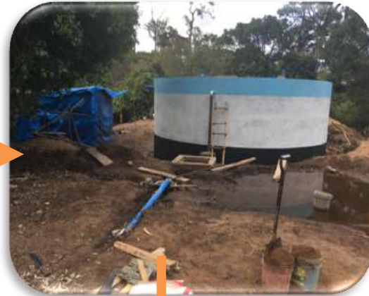
90 m 3 storage tank
