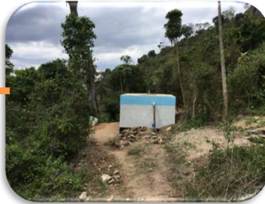
2Nos-15m 3 Break Pressure Tank
