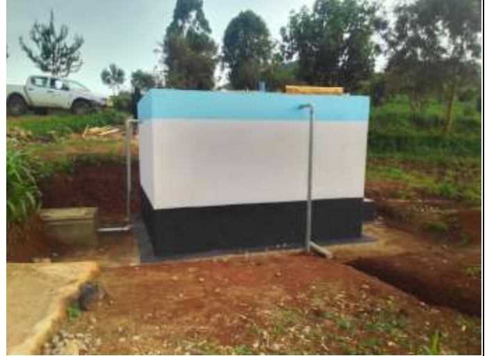
The 15m 3 storage tank for Mkatoni(2 DPs)
